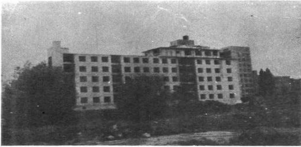
Structural design for apartment building, Roselawn Avenue, Toronto, Ont., by Z. Przygoda, consulting engineer.
